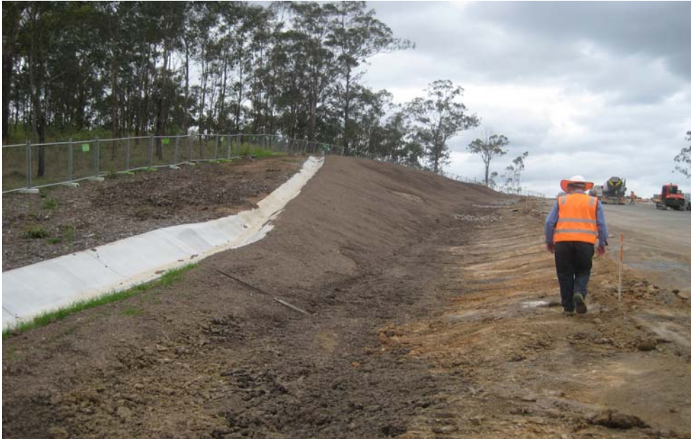
Figure D1-1: Site inspections are critical to review and monitor compliancy of construction works
