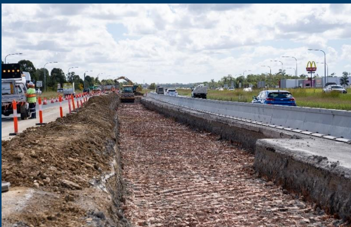
Earthworks underway for the new northbound Exit 152B from the Bruce Highway to the D'Aguiar Highway.
